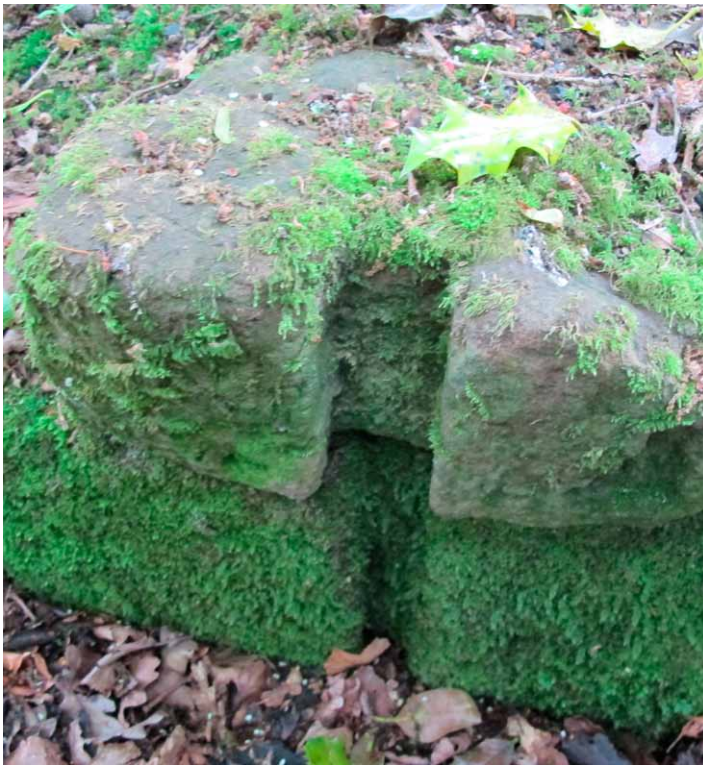
Fig 12. Slotted stones are often all that remains of water meadow sluices. They are difficult to date without evidence from other sources, though later sluices were often brick-built.
