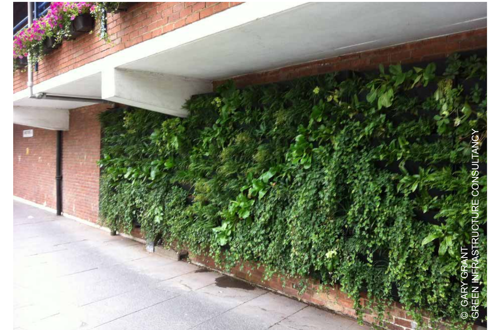
Figure 3. Vertical rain garden installed on social housing in London.
